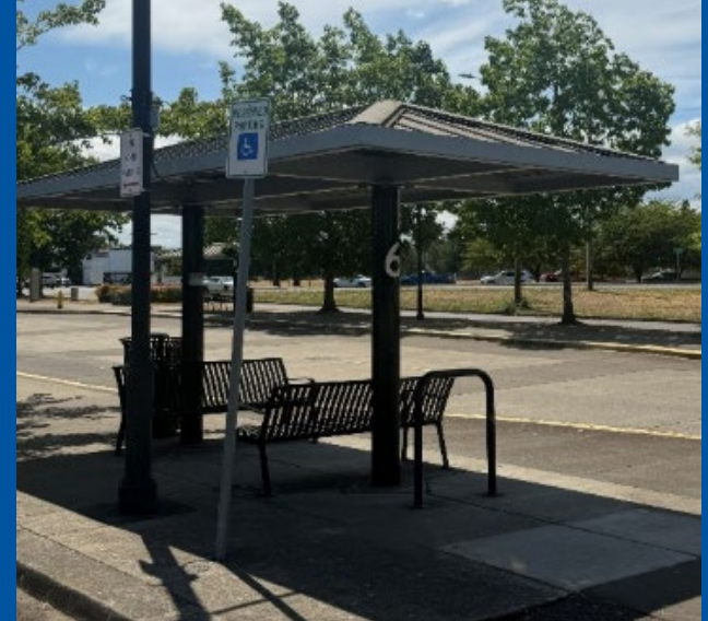
Shelter #6: No Visible Signage
